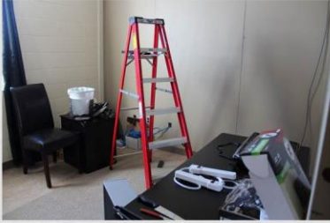
Monitor Room (being re-wired)
